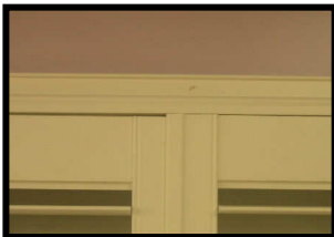
Once you have installed the panels, and they do not line up,
